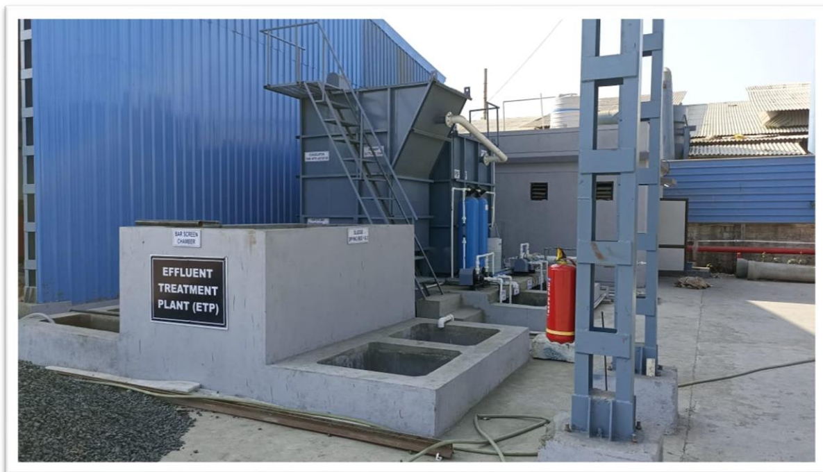
15 KLD ETP Plant at Gandhidham- Kachchh, Gujarat
